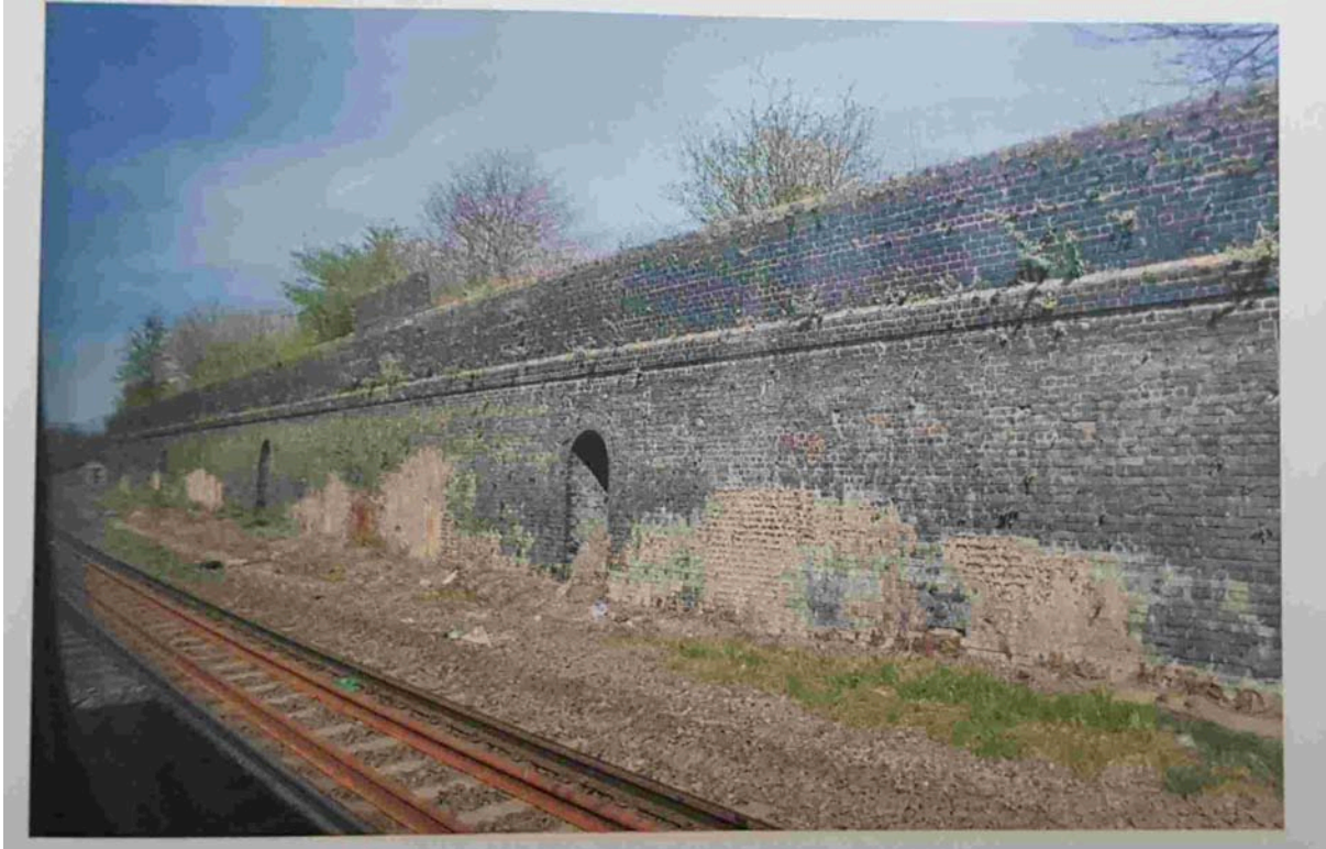
The railway retaining wall. Approximately 6m of retaining wall, topped by 2m of boundary wall. The heritage towpath is behind the boundary wall. The beaded section indicates ground level. Source: Manchester Bolton & Bury Canal Through Time.
