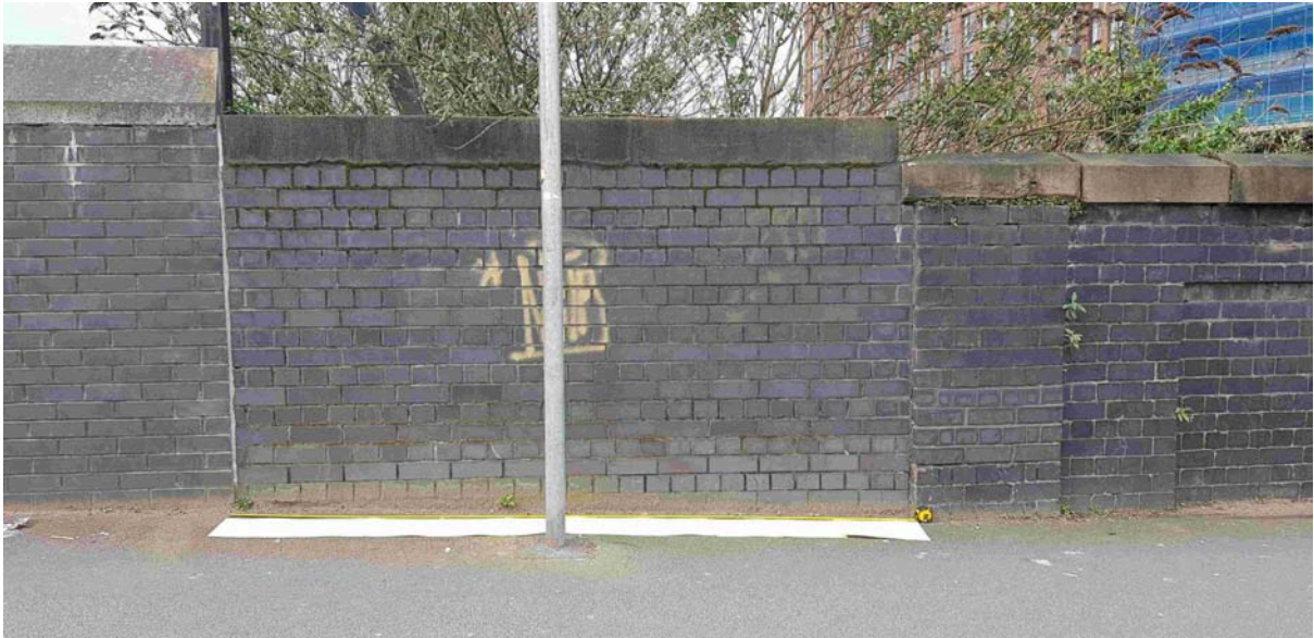
Contemporary MBBCS photo of the Towpath entrance. The yellow mat is 2.9 m wide The rest of the heritage canal parapet wall is an essential safety feature of any restored canal.
