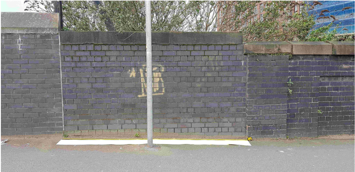
Contemporary MBBCS photo of the Towpath entrance. The yellow mat is 2.9 m wide The rest of the heritage canal parapet wall is an essential safety feature of any restored canal.
